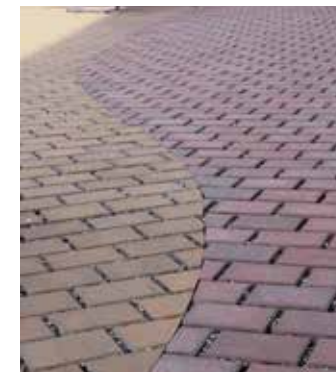
Figure 90: Permeable brick paving.
